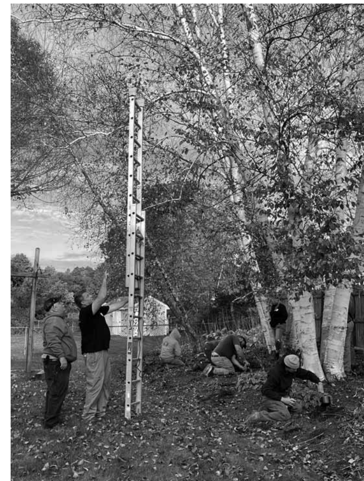
Participants install up-light fixtures on the ground as Jim Moreau and Eric Mitchell plan where to install down-lights within the birches.
