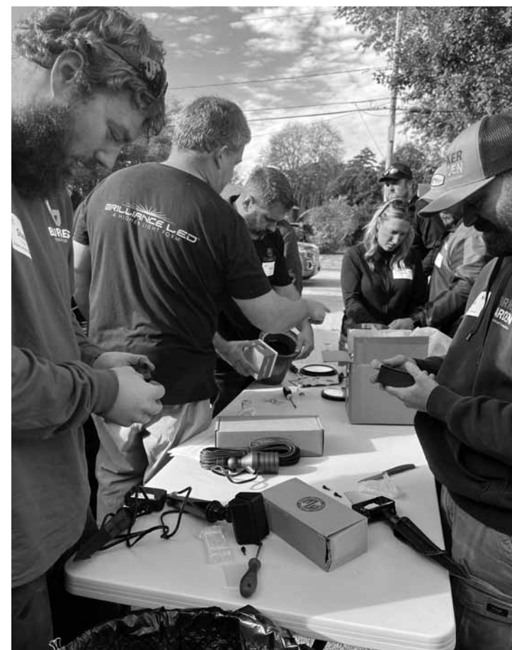
Participants assemble low voltage lighting fixtures in preparation for the lighting install.
