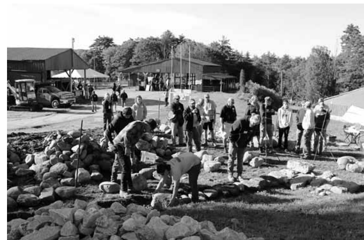
Attendees get hands-on experience working with members of The Stone Trust to construct a dry stone retaining wall.
