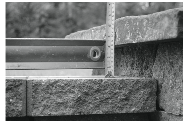
Here is a wall that has settled. You can see that the level is indicating a 1-inch dip because of poor base preparation.
